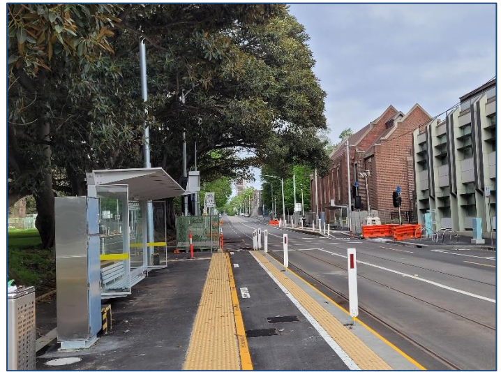
New twin platform tram turnback in Domain Road at ANZAC Station. – Image Geoff Mann
