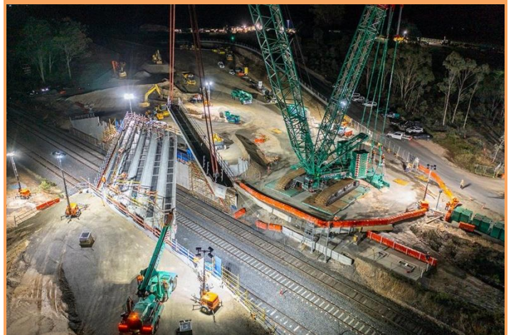
Final placement of new beams by ARTC at the Seymour = Avenel road overbridge between Seymour and Mangalore to provide double stacked container clearance for Inland Rail freight trains (Stage – 1) travelling between Melbourne – Albury – Wagga – Junee – Illabo – Stockingbal and Parkes. Photo – ARTC
