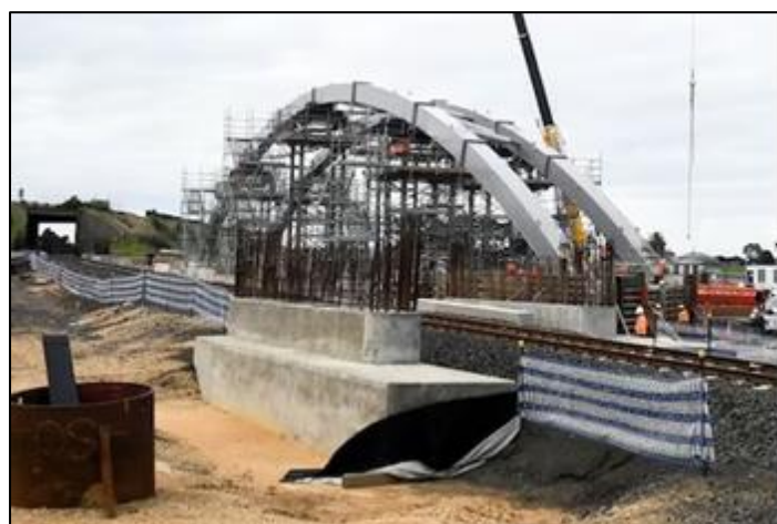
Late August 2023 and the new single track rail over road bridge has been placed into final position. - Photo Rail Projects Victoria
