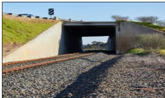
Existing Kilmany two lane road over rail overpass at Kilmany - Photo Rail Projects Victoria
