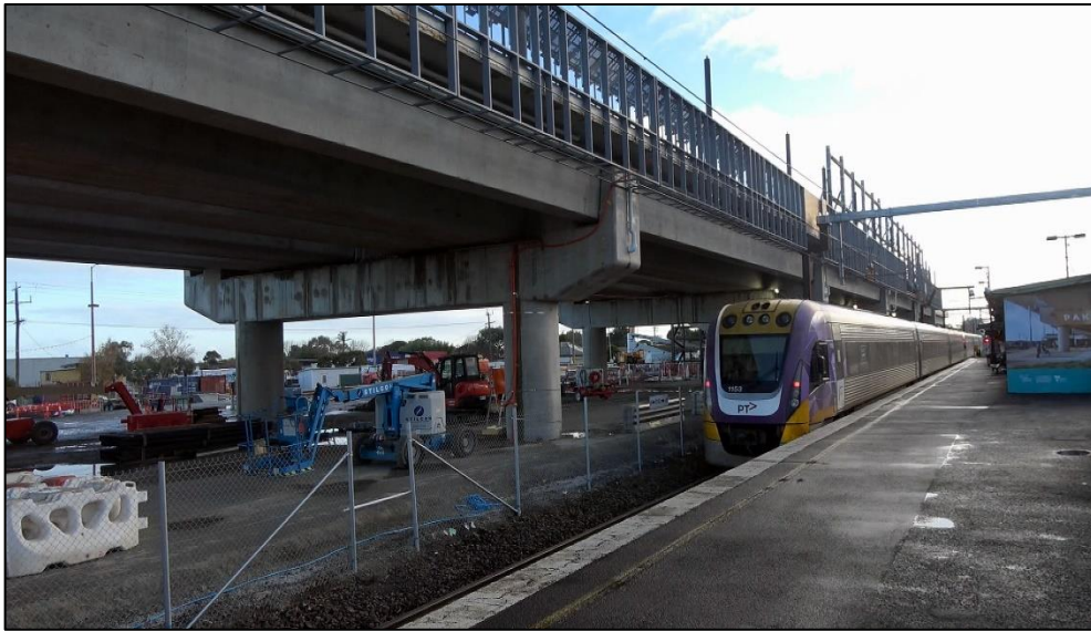
New overhead station taking shape at Pakenham, with an Up Traralgon Vlocity at the existing ground level Up platform.
