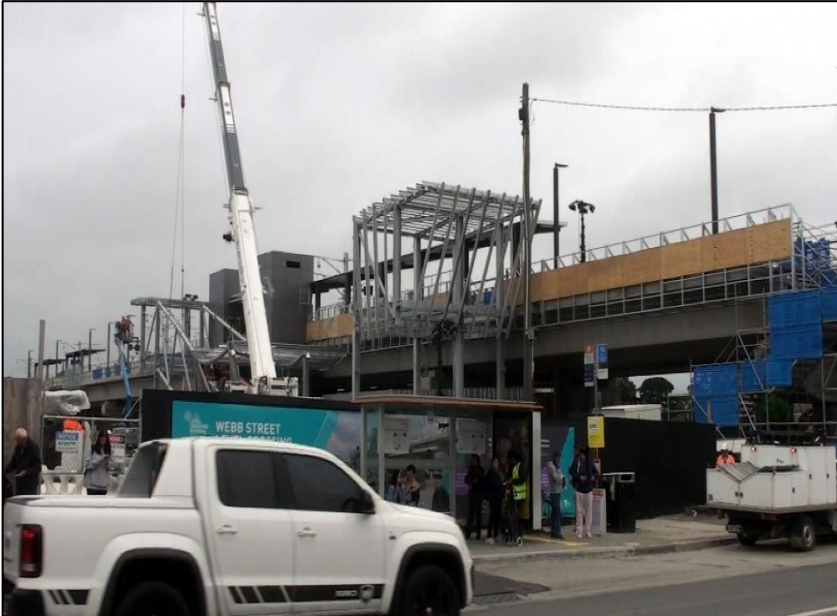
New elevated station at Narre Warren with steps, taking shape. Photo – Jonathan Scutt
