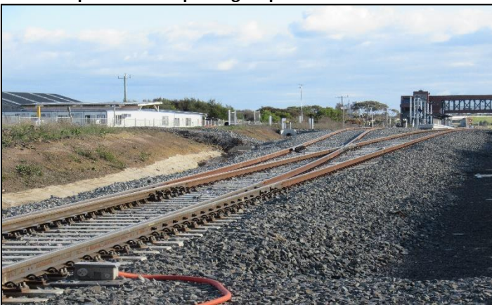
Also commissioned late May three position signalling and CTC control of signalling between Waurm Ponds station and Warncourt Loop on the Down side of Birregurra station.
