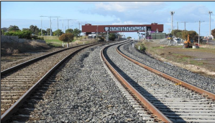
Finally completed and commissioned late May, 2022 the second platform and passing loop at Waurm Ponds station.
