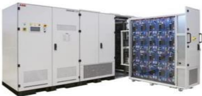
Innovative energy storage system as installed on the Hurstbridge line between Wattle Glen and Eltham.
